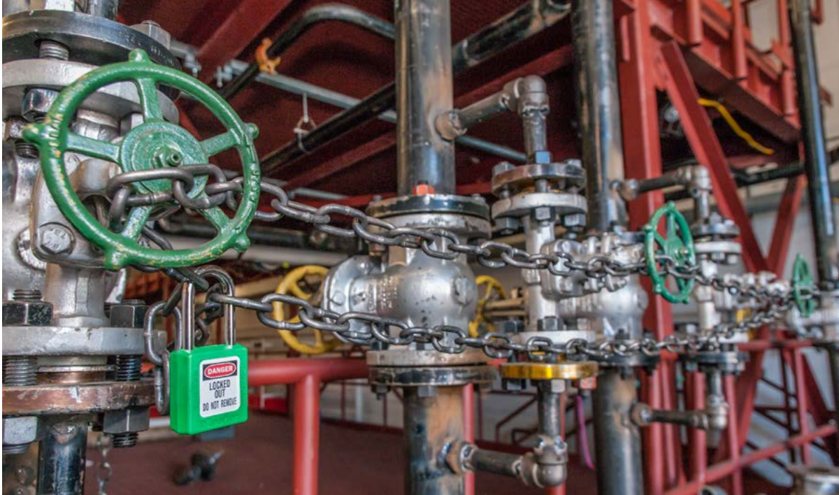
Figure 3 — Chains used to lock out valve handles
